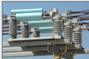
System Protection Equipment
