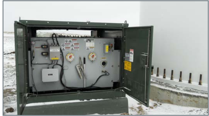
▲ Padmount switch installed outside the wind tower.
