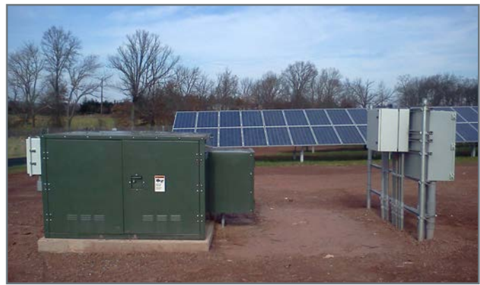
▲ Padmount switch installed in a solar application.
