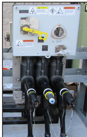
▲ For solid dielectric switches, all voltage sensing components are built into the epoxy module.
