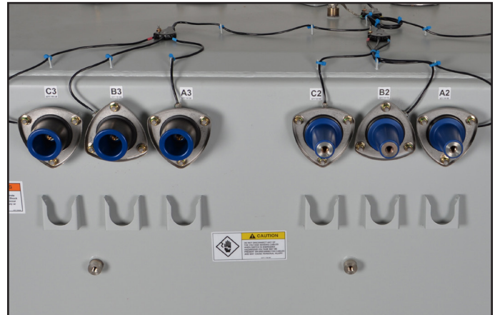
▲ Voltage sensing bushings mounted on a SF6 switch.
