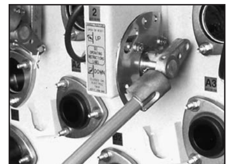
▲ Fault interrupter operating handle.
