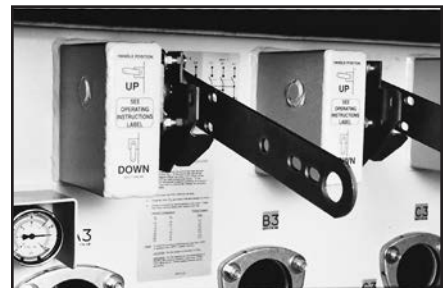
▲ Single phase interrupter operating handles.
