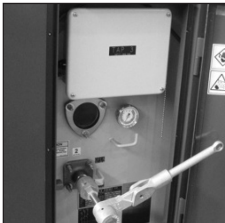
▲ All load break switch operators are located on the side of the switch.
