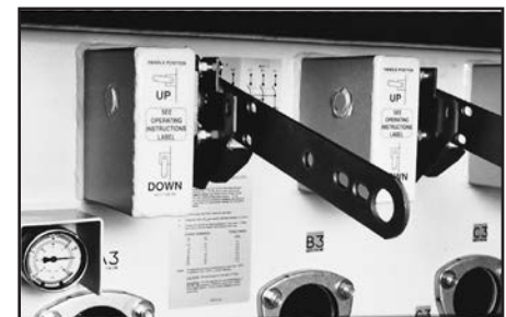
▲ Single phase interrupter operating handles.
