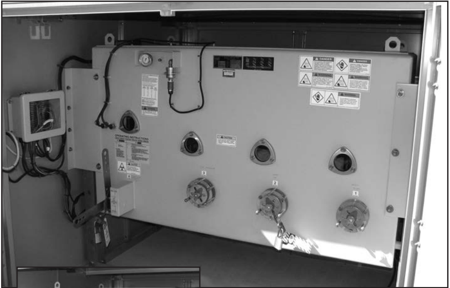
▲ Front and back view of a padmount PNI-43L with rotary style load break operator.
