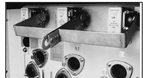
▲ Three phase interrupter operating handle.
