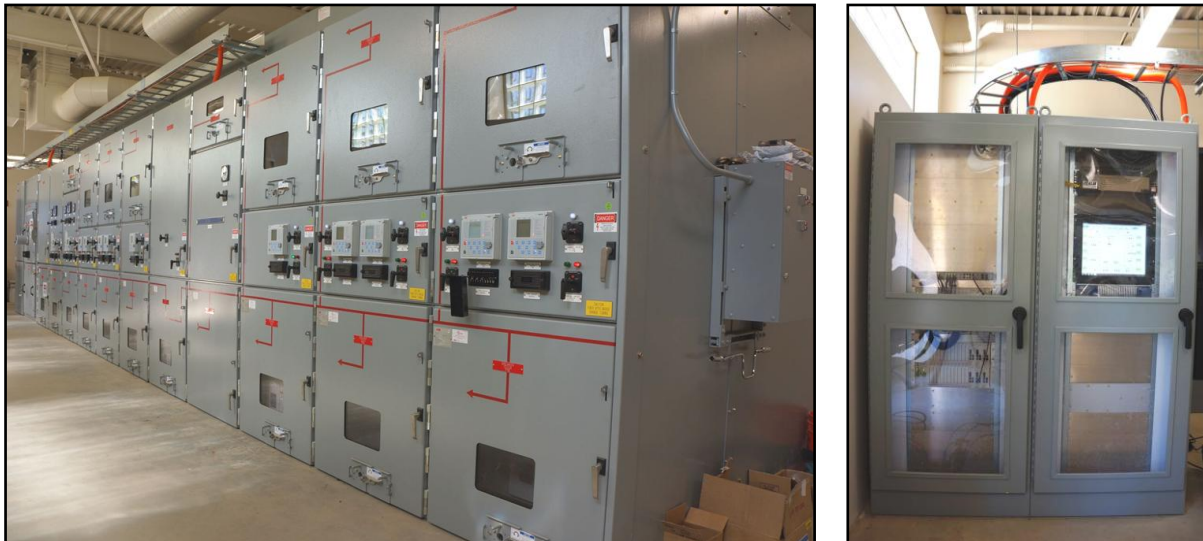
Figure 9: 12kV metal-clad switchgear lineup and control cabinet racks in switchgear control building
