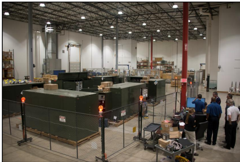
Figure 12: Factory Acceptance Test for complete automation solution
