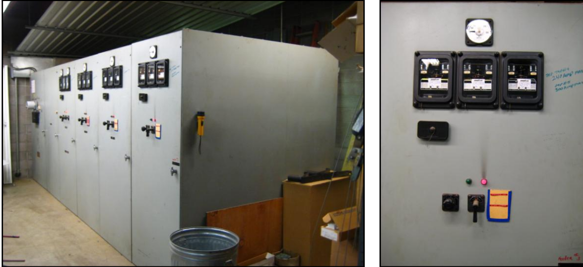
Figure 2: Old 12kV main and feeders breakers with relays
