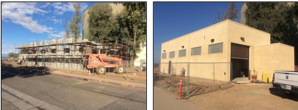
Figure 5: New 12kV switchgear building
