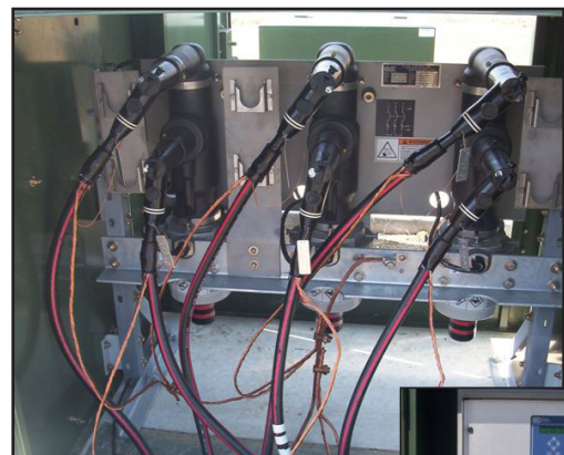
Photo above shows the recloser compartment access for cable connections.
