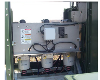
Recloser operator compartment
