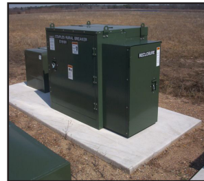
Padmount Viper-ST recloser
