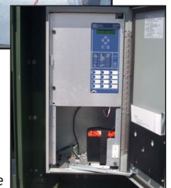
The SEL 651-R control is housed within a separate enclosure on the side of the recloser.
