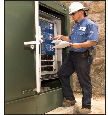
Control enclosure on the padmount switch showing three SEL-451 relays.
