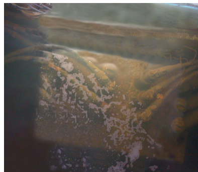
Top operable switch after submersion in water.
