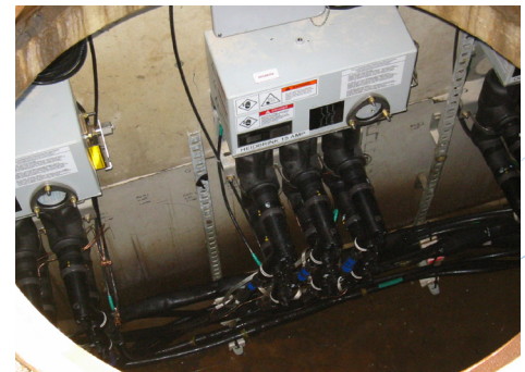
Solid dielectric switch installed in vault.
