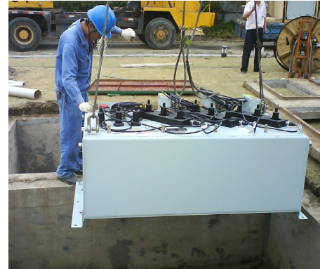
Submersible switch installed in a small, underground vault, subject to flooding.
