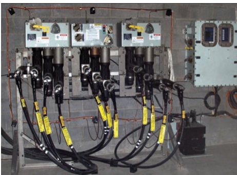
Three-way, solid dielectric, automatic transfer switch with submersible control cabinet and potential transformers.
