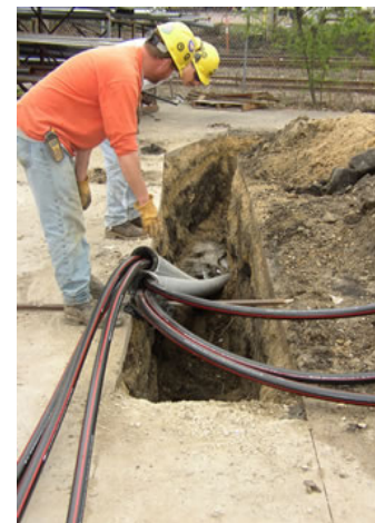
Underground cables can be direct buried or installed in conduit to switch locations.
