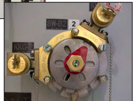
▲ Load break multi-position switch operator with keylocks.
