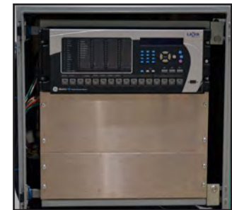
▲ GE F60 feeder relay
