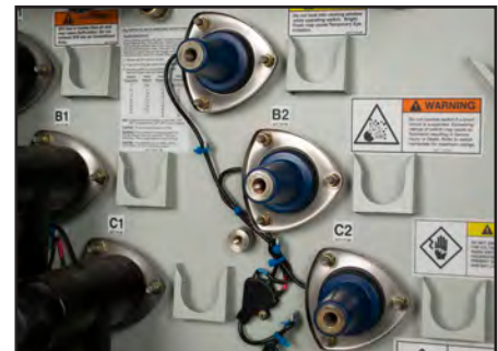
▲ Voltage sensing bushings mounted on a LPFI switch.
