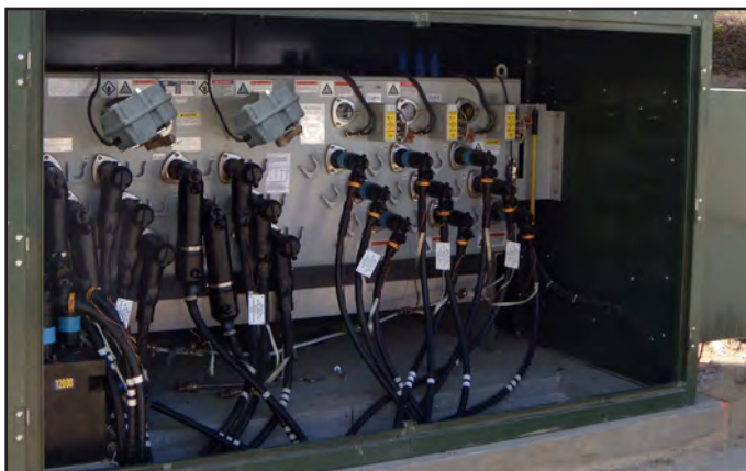
▲ Motor operators installed on a G&W automatic transfer switch.
