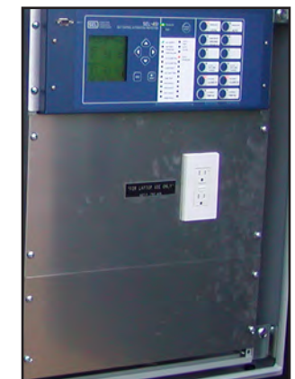
▲ SEL-451 mounted in NEMA 4 enclosure with convenience outlet.
