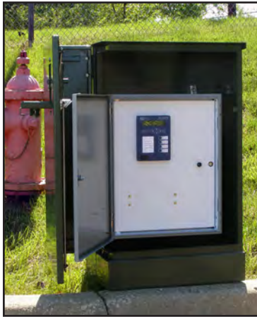
▲ Low profile curbside pedestal enclosure.
